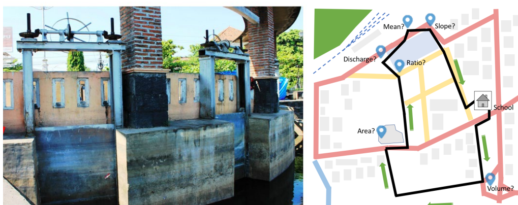
Figure 2. The task of the floodgates of Semarang Old Town in the Old Town Route
